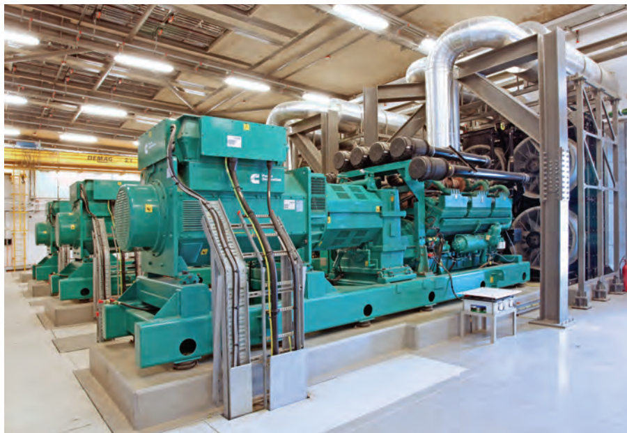
40 MVA MVA Standby Power at Muscat International Airport and Salalah Airport.
